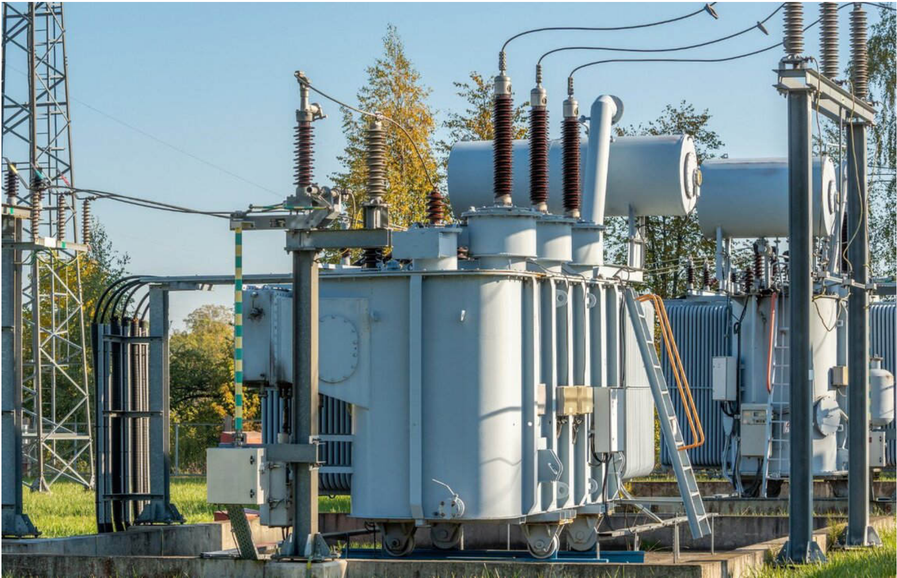
E-REDES transformer included in the Analytics4Assets project – AI-Driven Asset Management
