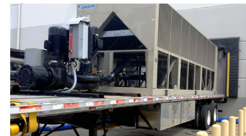
Air-cooled chillers installed at a data center in Texas
